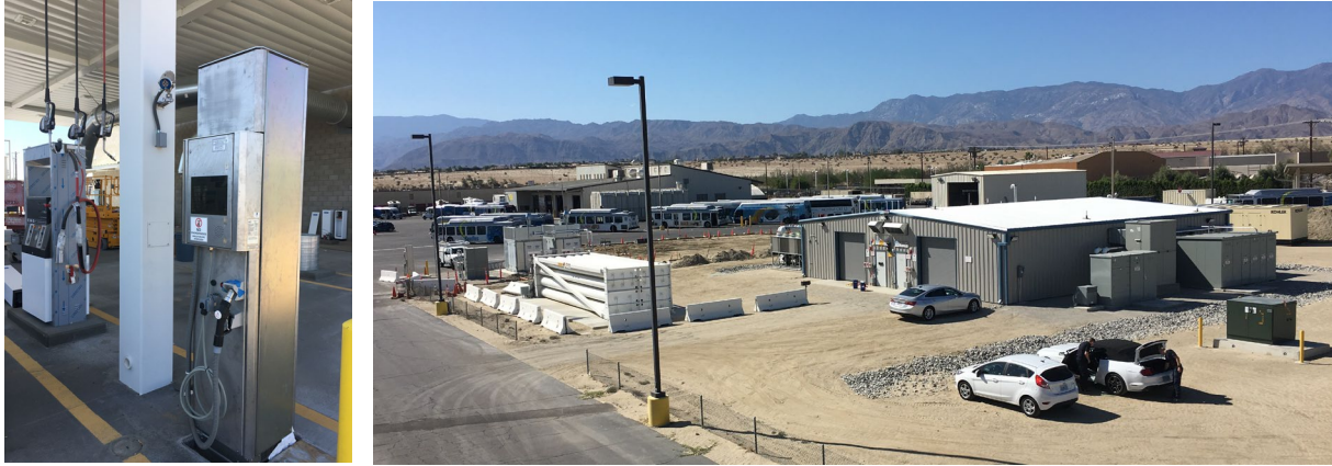
Figure 3 – Station photos. On left, hydrogen dispenser integrated into new CNG island. On right, panorama of full station.
